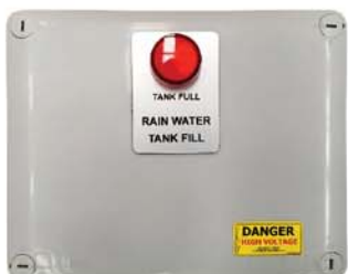
Waste Tank Alarm
